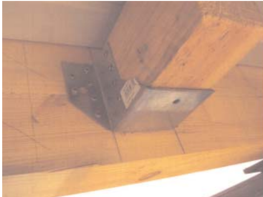
Photograph of the sample subjected to the test: Detail of the connection between the lower cross-members and longitudinal beams.
